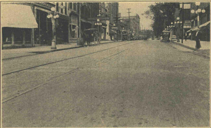
Figure 93. Waterbound Macadam Pavement—Having Same Traffic and Treatments As Surface Shown in Figure 92, After Six Years Maintenance
