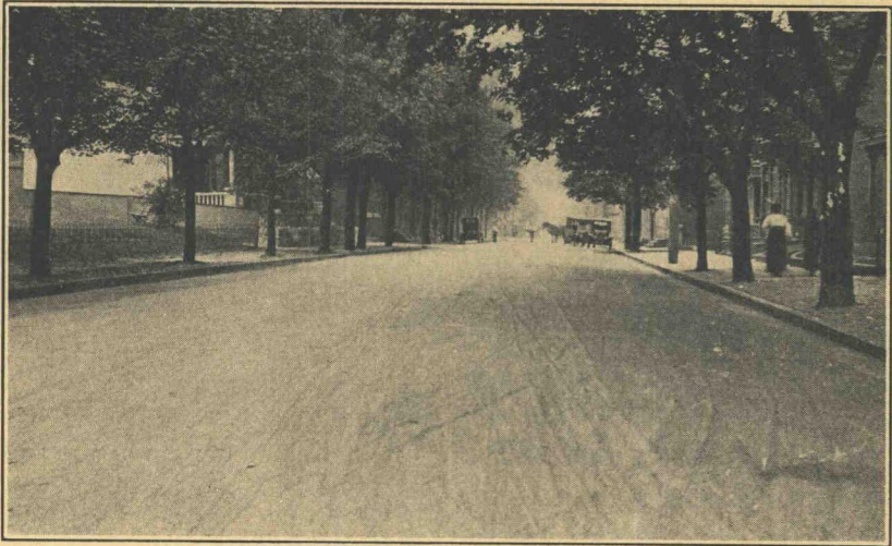
Figure 96. Bituminous Macadam Surface About Four Days After the Application of Light Bituminous Material and Sand
