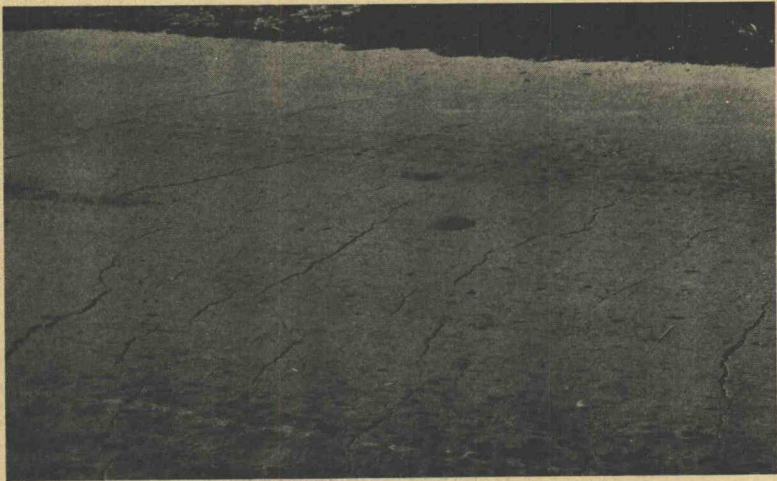
Figure 5. Early Cracking in Concrete Pavement Eliminated by Placing Tar Paper on Subgrade. (Photograph furnished by R. W. Crum.)
