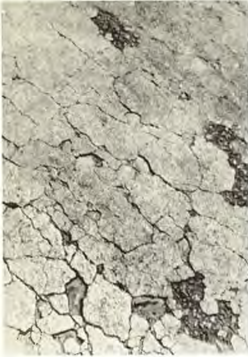
Figure 2. Failure of concrete on US 1 in Dumfries, Virginia.
