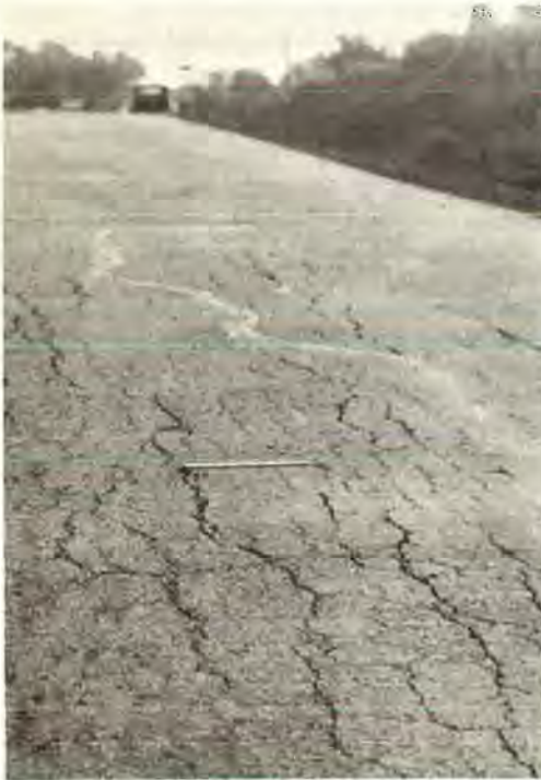
Figure 1. Cracking of concrete pavement in Georgia.
