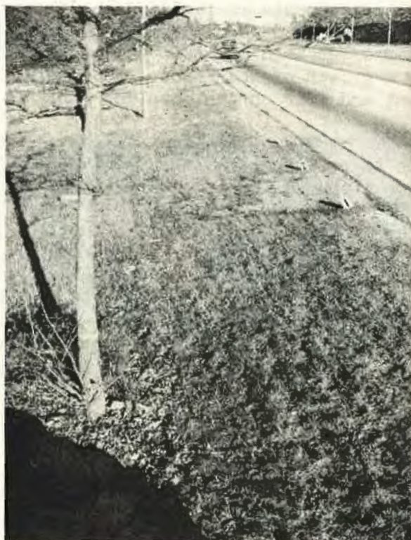
Figure 8. Project 8444 (11/18/47) Beyond location 3 (see cut) shoulder untreated; 2 to 3 cinder shoulder; 1 to 2 stone shoulder; foreground stabilized soil shoulder
