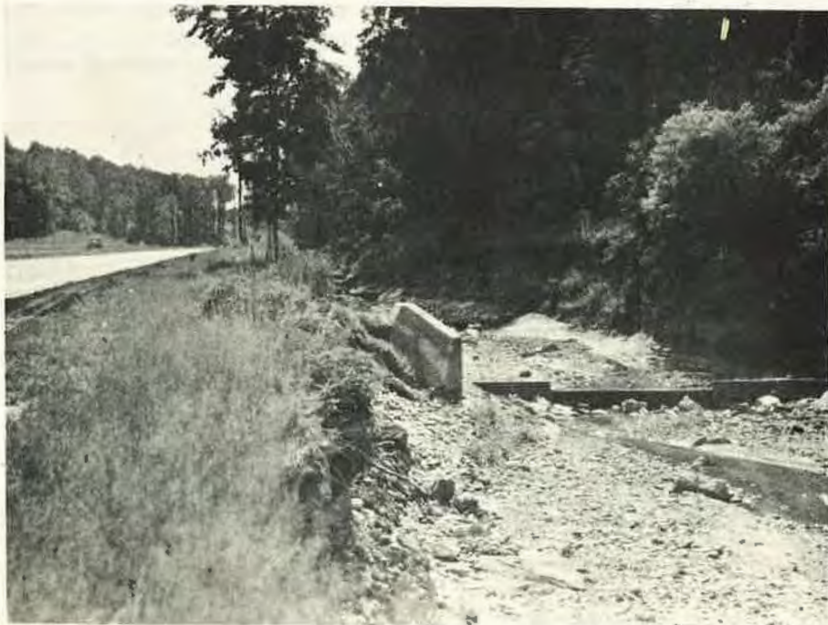
Figure 19. Another Stream Channel Paralleling the Same Highway. Stream banks as well as the stream bed will require protection against increasing volumes of surface water resulting in changes of land use on adjoining watershed lands.
