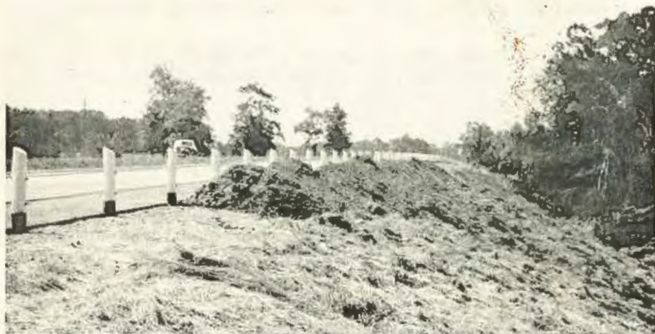
Figure 20. An Easy Well-rounded Slope Being Mulched Immediately Following Construction of a New Highway. A light covering with soil over the mulch will be followed by seeding.
