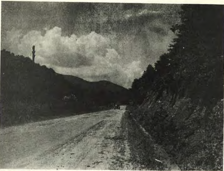
Figure 5. One of the Earliest Federal-aid Highways Constructed in the 1920 Decade. Note steep side slopes and heavy erosion resulting in blocked drainage. Erosion can hardly be controlled since vegetation cannot be established or maintained on such a cross section.
