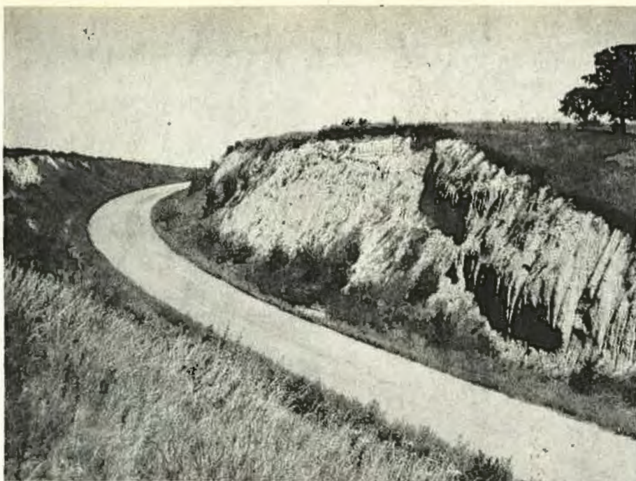
Figure 8. An Old Model State Highway With Clogged Drainageways Resulting from Erosion of Steep Angular Slopes. Before reconstruction.
