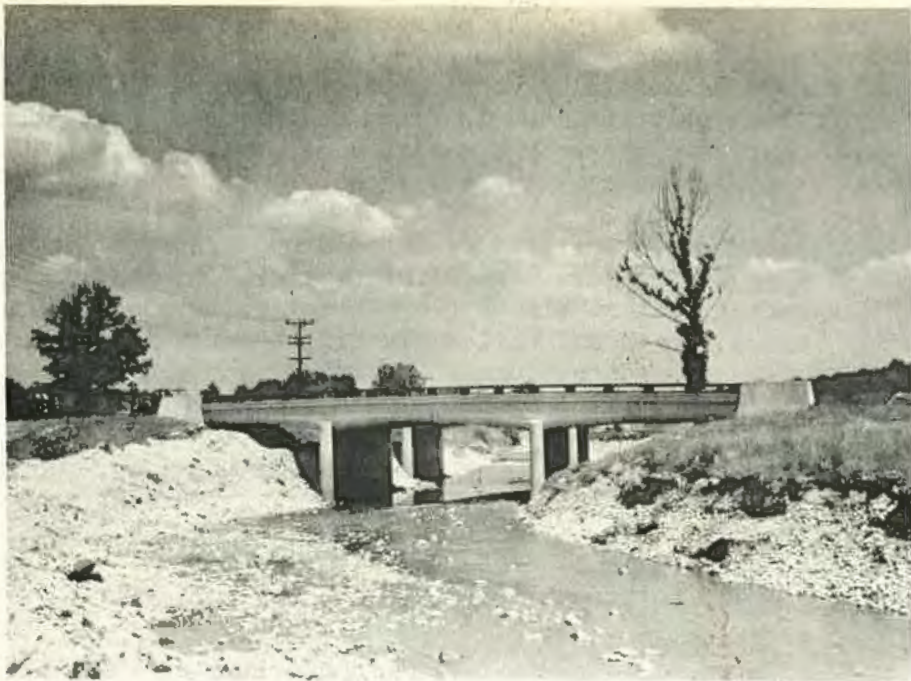
Figure 18. A Bridge Shown at Left in Figure 17. Note heavy erosion resulting from increased run-off on paved city streets draining into the stream watershed. Riprap, combined with willow bank protection will now be necessary to protect bridge embankments and keep the channel open. Such erosion control work can be done most economically when it is part of the original highway design and construction.
