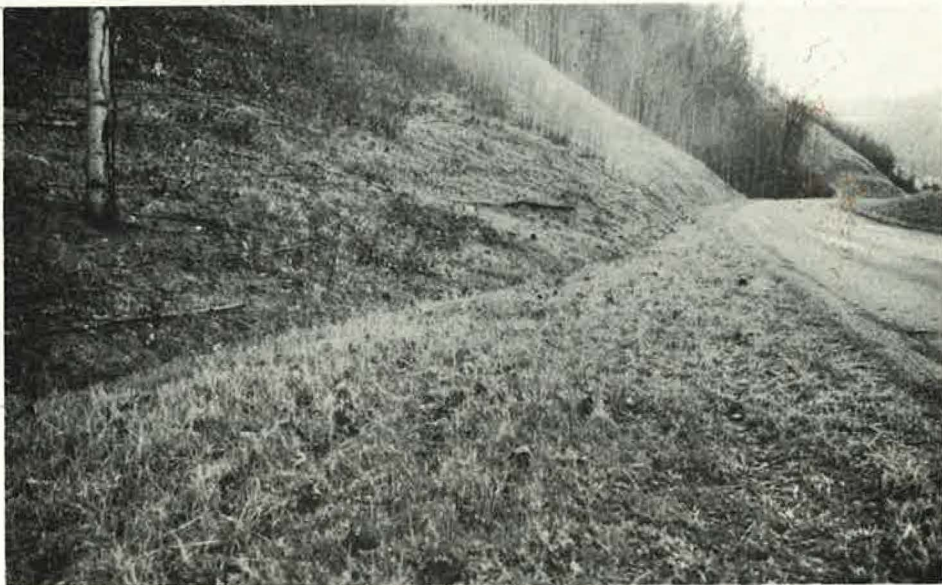
Figure 18. In a Well-Designed Transition, Gutter is Led Away From Fill. Erosion Damage to Slopes is Prevented By Including Seeding and Mulching in Grading Contracts.
