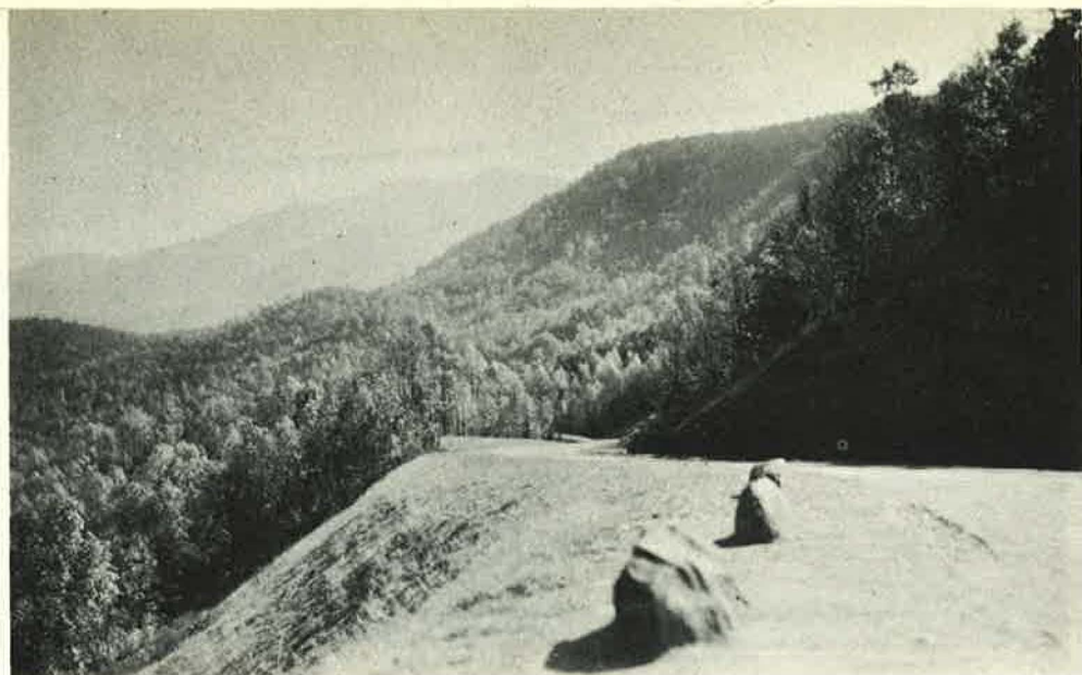
Figure 7. The Hillock in Middle Distance is "Daylighted" or Cut Off Flush With the Grade. Note Seeded 1\frac{1}{2} to 1 Fill Slope in Foreground.
