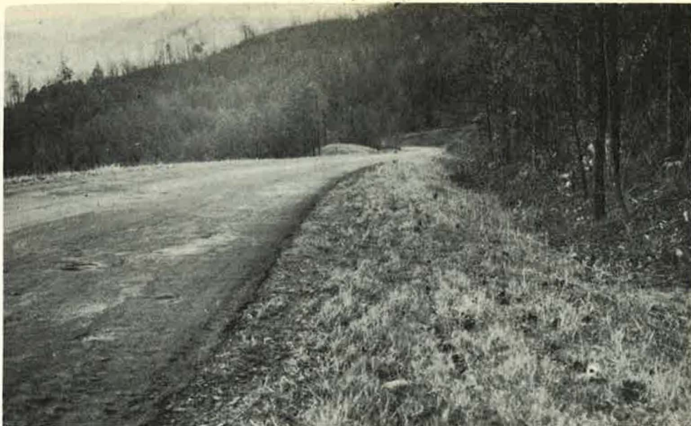
Figure 9. Small Pocket Fill Right Foreground. Filling up Such a Small Pocket Often Obviates Need for Culvert.
