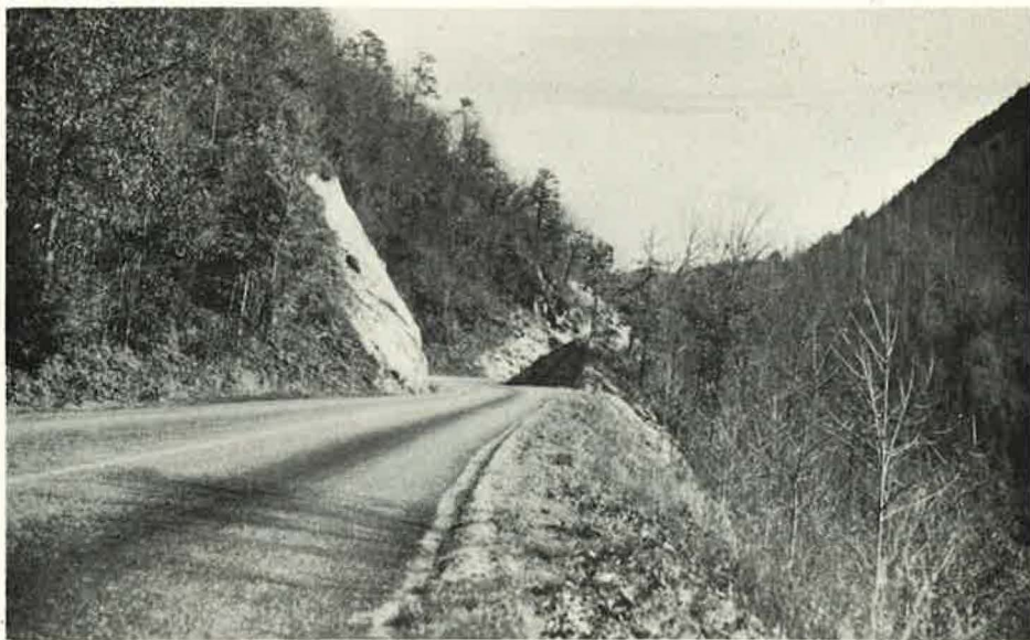
Figure 2. Removal of Residual Hillock Often Increases Sight Distance.
