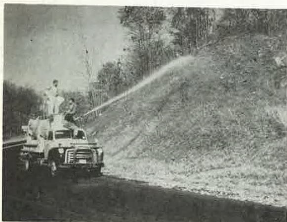
Figure 12. Connecticut State Highway Department spray equipment is used to seed, fertilize, and spray resin simultaneously.
