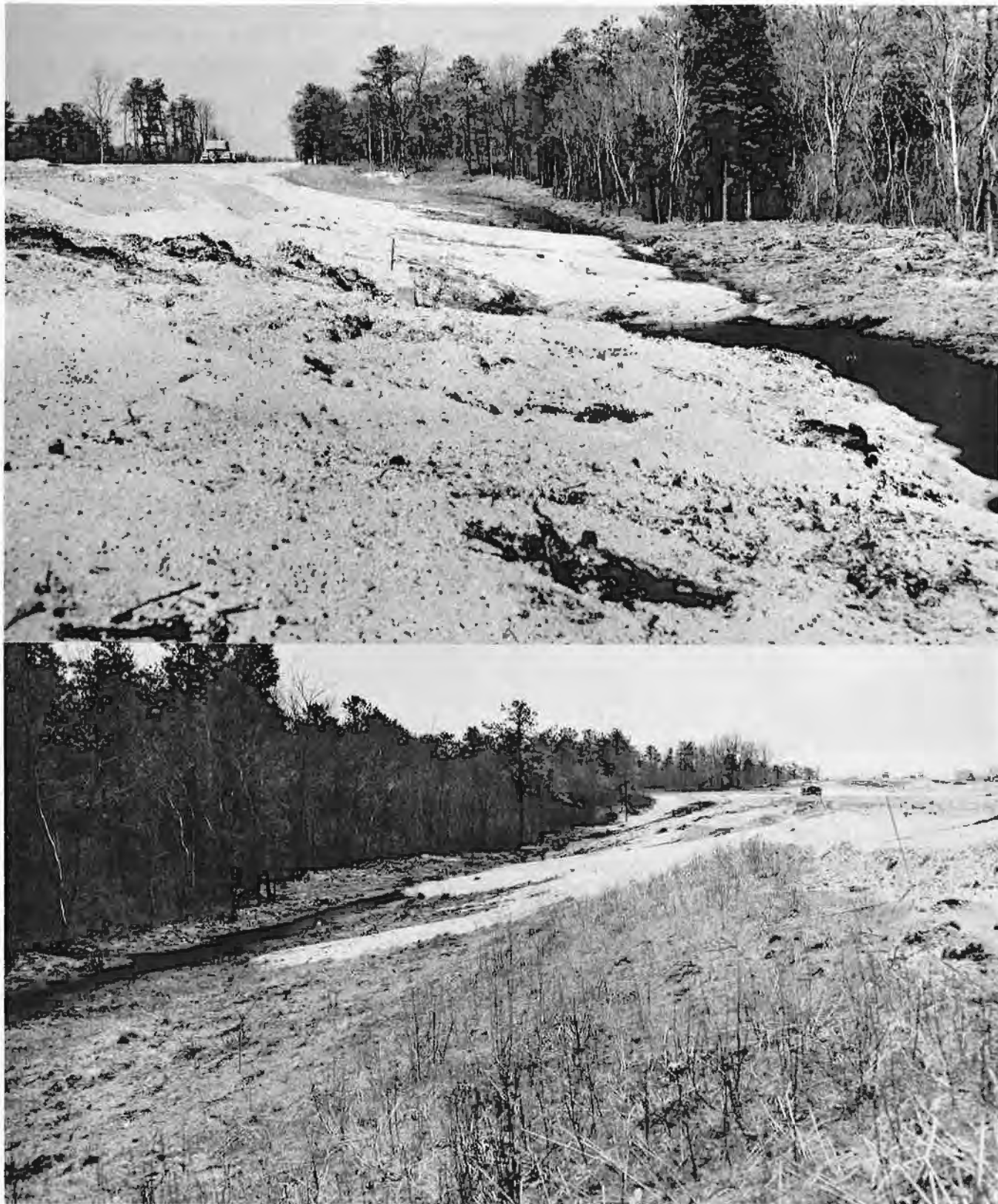
Figure 6. Contrast between finished surfaces which have been seeded and mulched as compared with adjacent areas left exposed. Note how eroded material has clogged drainage, necessitating additional grading.
