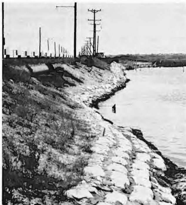
Figure 2. Riprap slope protection is used where salt water and tidal currents prevent growth of vegetation.
