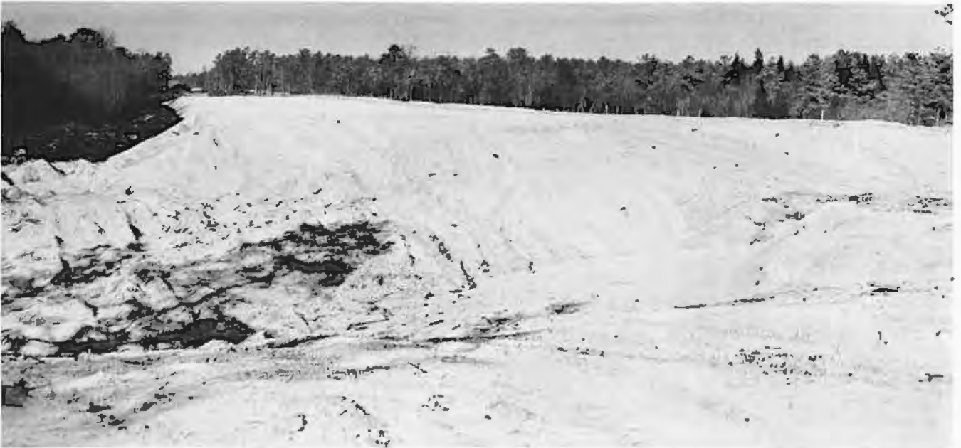
Figure 3. Early stage of construction showing the type of sand fill used in all areas shown in Figures 4, 5, 6, and 7. Note storage piles of native peat excavated as unsuitable fill material, at extreme left.
