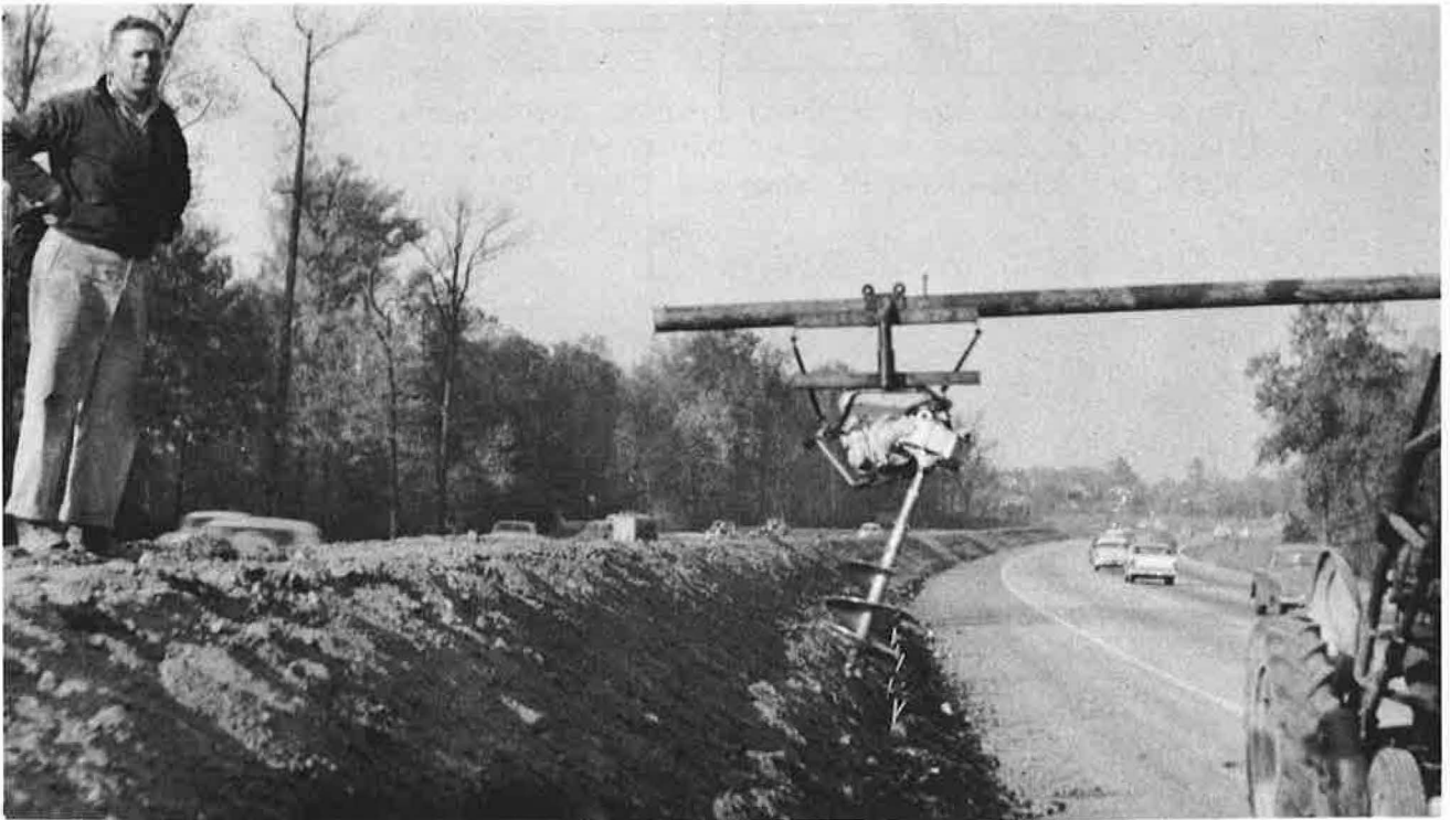
Figure 11. New Jersey's Garden State Parkway, showing mounding of median and planting of the mound with Hall's Japanese honeysuckle. Power auger was used to dig the planting holes for the honeysuckle; autumn, 1956. (Courtesy New Jersey State Highway Department)
