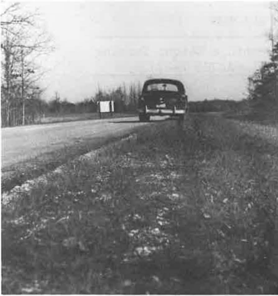
Figure 3. Stabilized shoulder on 2A11 portion (Alabama) after final compaction and one full growing season. Photograph taken during winter. Tire track from car is only faintly visible on super-saturated stabilized shoulder.
