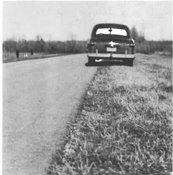
Figure 6. On Project LH6-1J9-2All. Close view of turf on stabilized shoulder during winter months following final compaction and one full growing season. Shoulder is thoroughly saturated, but only a slight tire track is evident immediately behind the car.
