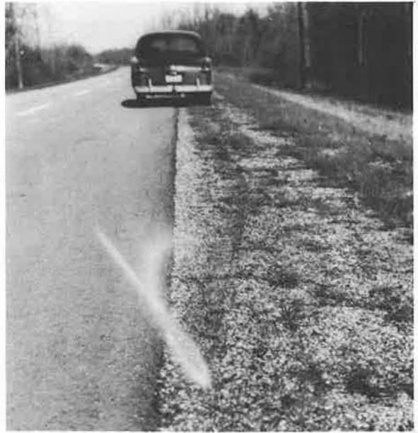
Figure 4. Stabilized shoulder on 2A11 portion (Alabama) after final compaction and one full growing season. Photograph taken during dormant winter months. The "ghost finger" inexplicably points to the tire mark, which is only a slight indentation on the super-saturated stabilized shoulder. This is one of a few places where the grass developed poorly; numerous quail flocked to this area and may have eaten all the seed.
