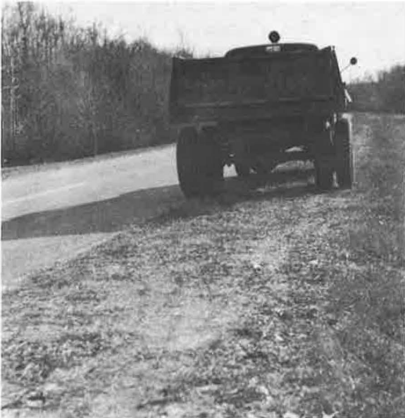
Figure 5. On Project LH6-1J9-2All following final compaction and one full growing season. Note supersaturated stabilized shoulder after several passes with empty maintenance truck. Grass is in winter dormancy.
