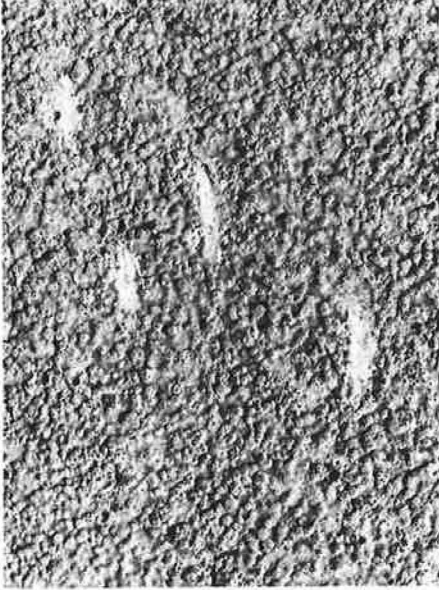
Figure 4. Closeup of tire stud gouge marks in a beaded paint line.
