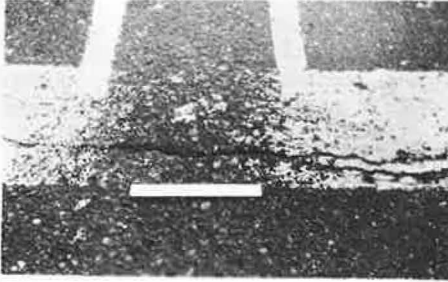
Figure 1. Wheel track area after 7,027 repetitive crossings of an automobile equipped with four studded tires (courtesy of the Minnesota Department of Highways).
