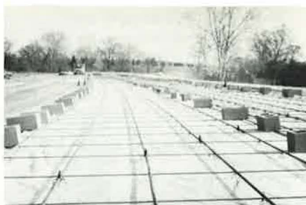
Steel tubing (strand enclosed) with grout fittings in place on 2-foot centers over No. 4 reinforcing bars on 2½-foot centers. Concrete blocks are to prevent the wind from lifting the double layer of polyethylene sheeting.
