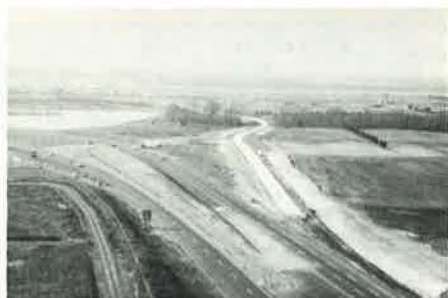
Aerial view of the prestressed pavement looking west. White polyethylene stands out in high-way right-of-way.
