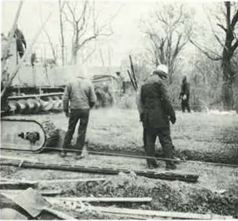
Steam rising from the fresh concrete. Air temperature was 35 F, and the concrete temperature was 55 F.
