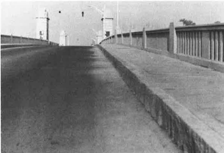
Figure 6. 112th St. Bridge, Troy, after repair; new roadway slab and steel grating on bascule span, new granite curbs, sidewalks repaired and protected by epoxy bonding compound covered with silica sand for traction, all concrete repaired and waterproofed.
