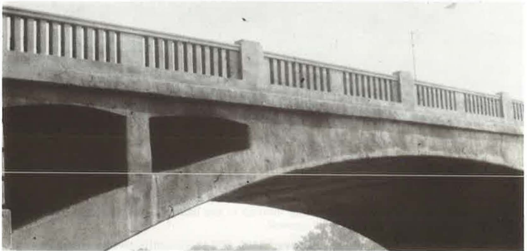
Figure 4. Railing after repair with gunite and waterproofing paint, 112th St. Bridge, Troy.
