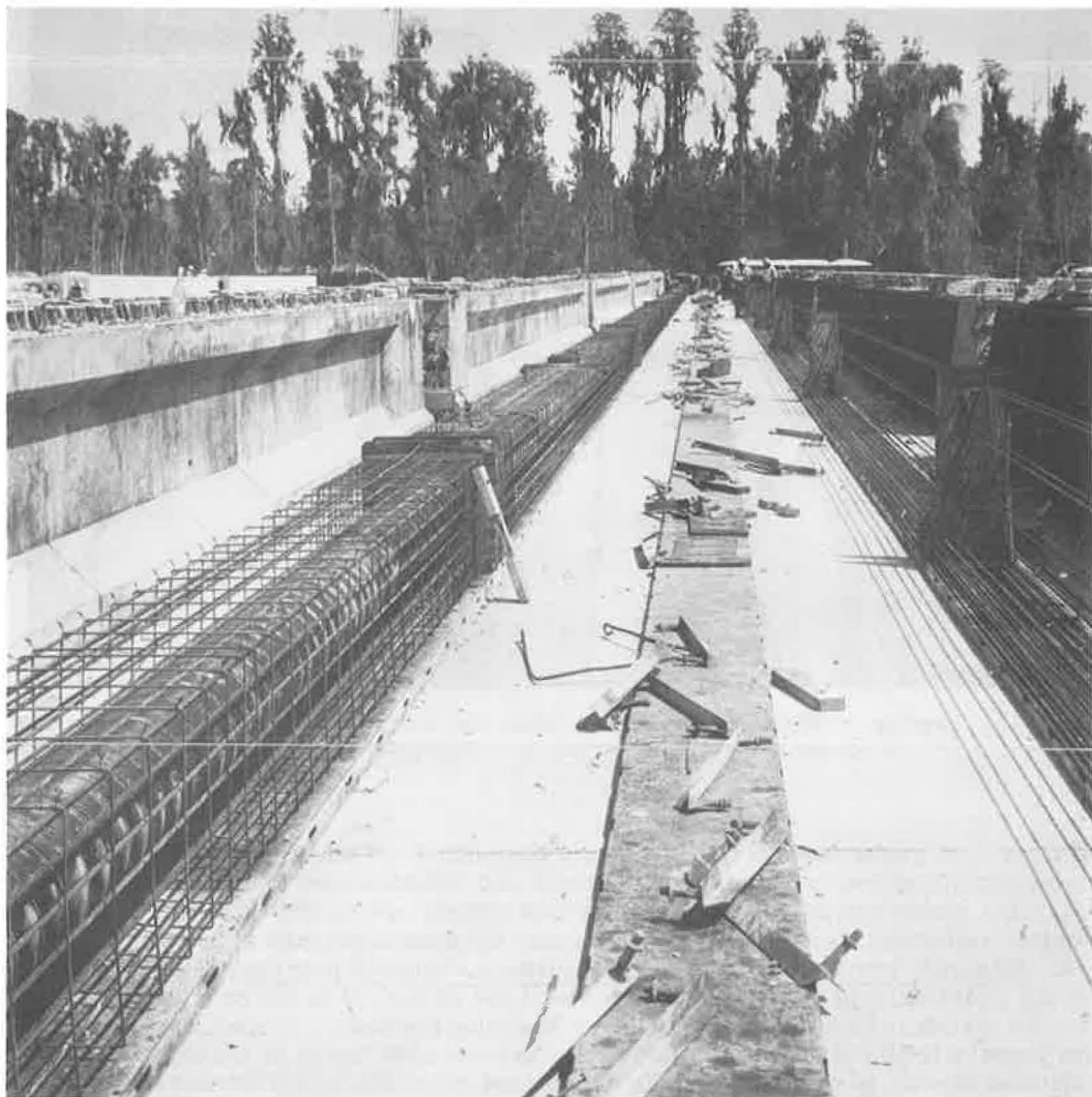
Figure 13. A line of finished girders with end blocks (left), and a line of forms for similar girders (right). Due to presence of end block, each beam must be formed up individually. Without end blocks forms are set up in one continuous line with sections permanently assembled in easily handled lengths.
