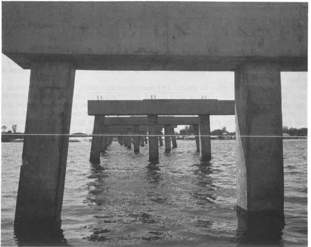
Figure 11. Four 24-in. square prestressed piles extend to provide pier columns for typical Florida crossing.
