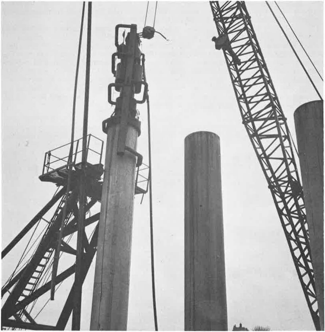
Figure 12. Driving pretensioned cylinder piles for a bridge in Tacoma, Wash.; 48-in. piles driven plumb to act as columns for piers.
