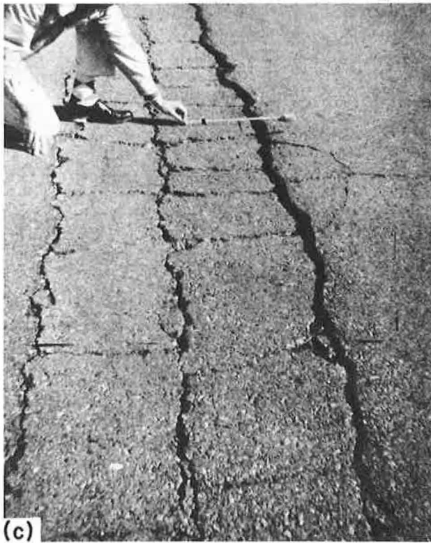
Figure 4. Typical progressive deterioration from shoulder cracking: (a) early shoulder cracking; (b) progressive cracking into driving lane; and (c) ultimate failure.
