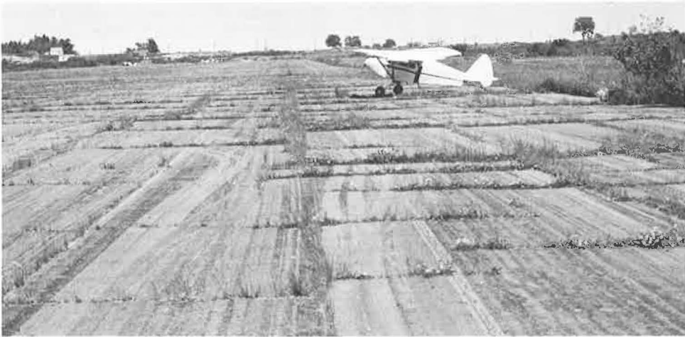
Figure 1. Eastport Airport before bituminous macadam overlay.
