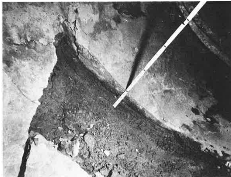
Figure 8. An 84-in. pipeline repaired by pressure grouting; several pipe sections were removed to observe grout distribution. Line has served 16 years since repairs were made and is in good condition.
