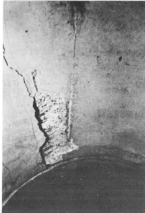
Figure 5. Concrete protective cover beginning to spall; can usually be repaired by chipping and guniting after sufficient passive soil pressures have developed to establish a state of equilibrium. Extreme cases may require pressure grouting to improve bedding conditions and lateral pressures.
