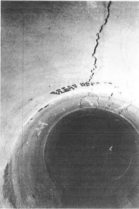
Figure 4. Longitudinal crack about 1/16 to 1/8 in. wide; easily repaired by chipping and guniting after sufficient passive soil pressures have developed to establish equilibrium.
