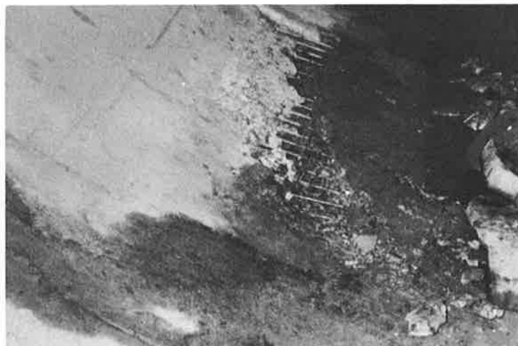
Figure 6. Advanced stage of spalling; note how reinforcement has pulled away from concrete wall. This 108-in. pipeline was repaired by pressure grouting through holes drilled at lower quarter points, after which new concrete protective cover was applied. Line has served 18 years since repairs were made and gives promise of a long satisfactory life.
