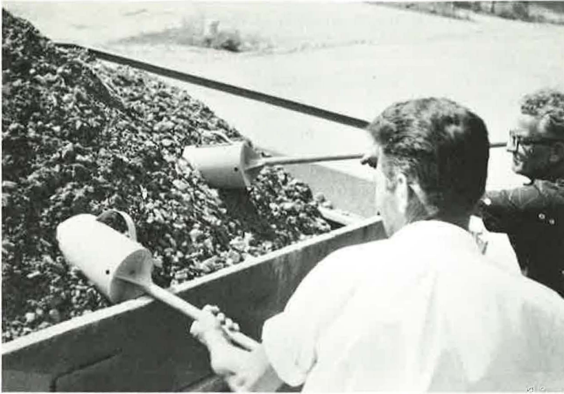
Figure 19. An aggregate used for construction of a stabilized aggregate base course was investigated in Series No. 5. The truck samples (after pugmill mixing) were secured with a sample thief. This device provided increment weights of approximately 15 lb each.
