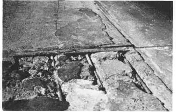
Figure 1. Concrete disintegration adjacent to an armored joint due to incompressibles in the joint.
