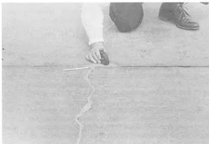
Figure 20. Crack repair in a rigid pavement.
