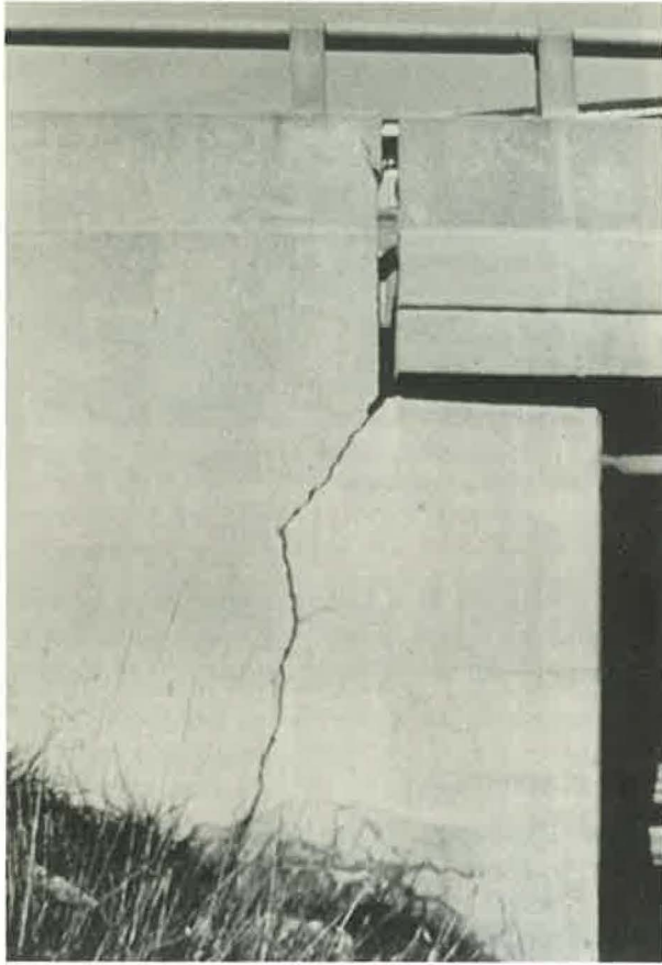
Figure 3. Abutment cracking due to pavement pressure.
