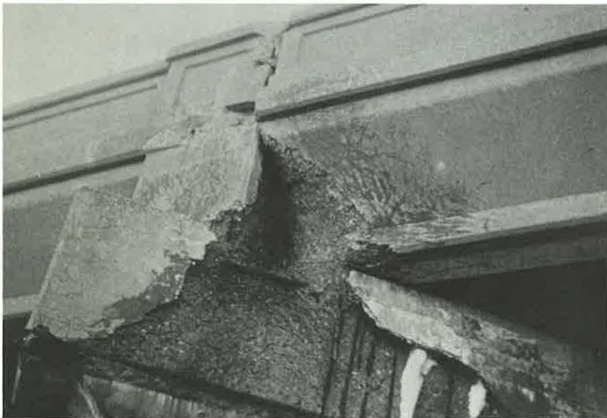
Figure 4. Concrete disintegration beneath an open bridge joint.
