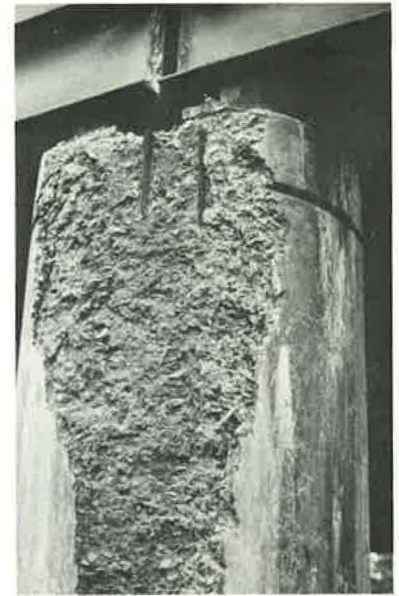
Figure 13. Salt and water damage to a bridge column beneath an open joint.
