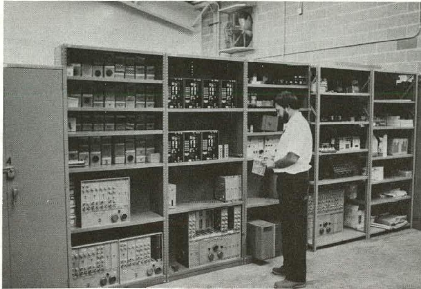
FIGURE 16 Spares stacked at a signal shop in Macon, Georgia.
