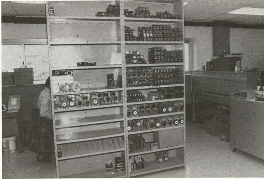
FIGURE 18 Electromechanical supply rack in Milwaukee containing dials, relays, and other devices. Units to the left are to be cleaned; those to the right have already been cleaned.
