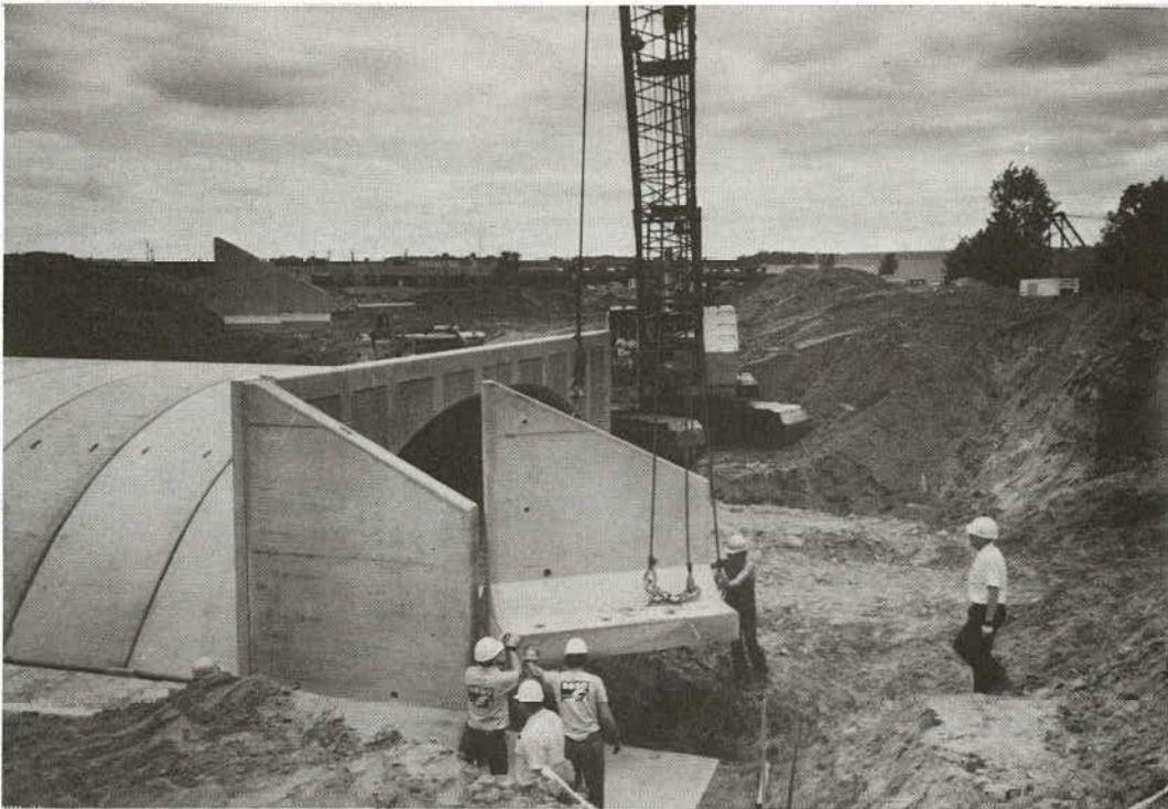
Figure 15 Precast wing wall is placed into position on site-cast concrete footing (Hancock Concrete Products photo).
