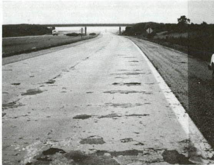
FIGURE 3 Severe D-cracking affecting most of the pavement slab.
