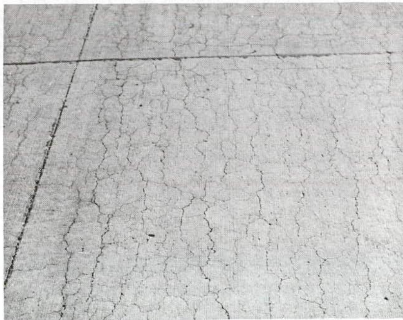
FIGURE 4 Map cracking caused by alkali-aggregate reactivity (9).
