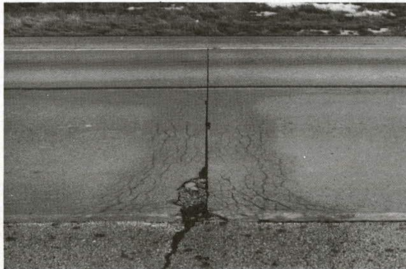
FIGURE 2 Development of D-cracking along a transverse and longitudinal joint.
