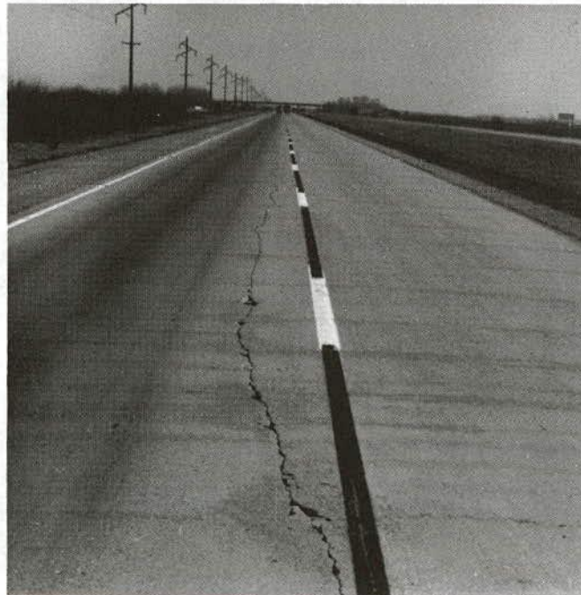
FIGURE 5 Staining or surface discoloration along cracks in a CRC pavement that often precedes surface D-cracking.
