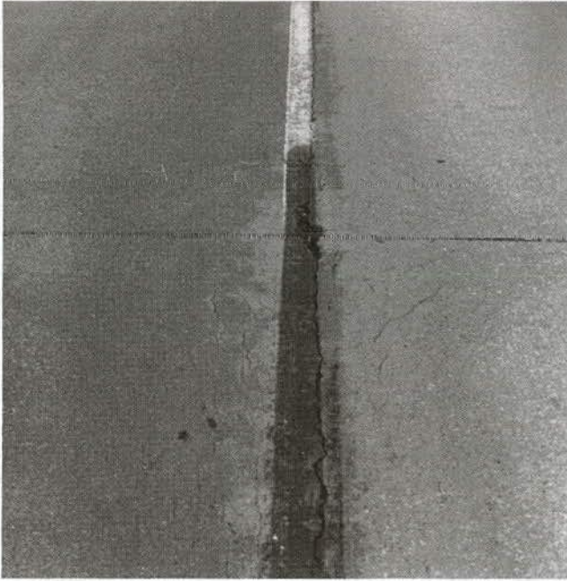
FIGURE 1 Initial appearance of D-cracking at intersection of transverse and longitudinal joint.
