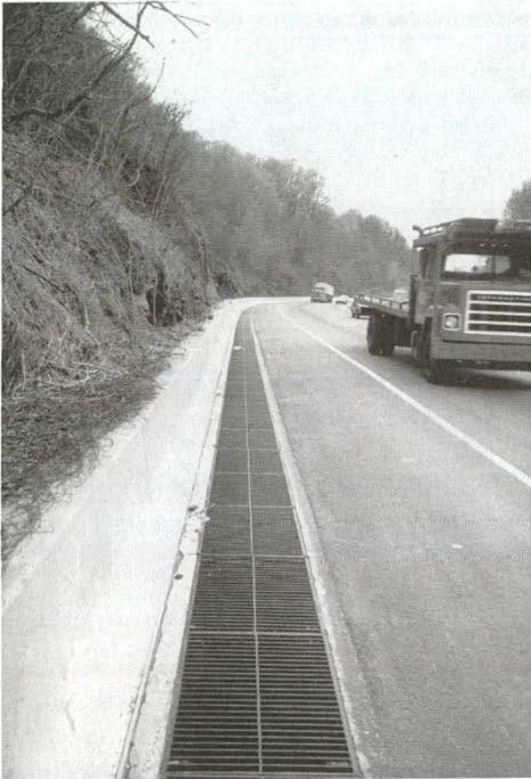
FIGURE D-11 Longitudinal surface drainage system installed on high side of superelevated curve to intercept groundwater and surface drainage from slope. This treatment prevents ice buildup during winter and was installed during I-4R upgrading of urban expressway.
