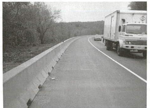
FIGURE D-12 Shoulder high side of superelevation of roadway rolled over in a well-rounded cross-vertical curve. Rain and/or snow meltwater will not flow down across travel lanes but back to concrete barrier, which is slotted to facilitate drainage. (Note concrete Jersey barrier used for outside guide rail in lieu of "W" beam to reduce maintenance on this urban expressway.)
