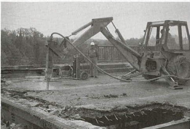
FIGURE 3 A hydraulically powered breaker being used to punch out the perimeter of a section of bridge deck.
