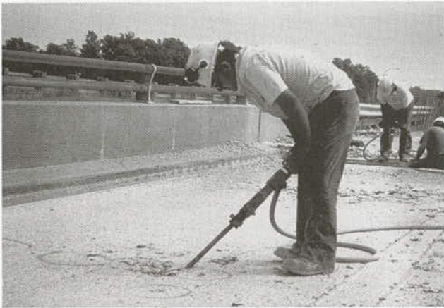
FIGURE 10 Use of a jackhammer to remove concrete to the level of the reinforcement.
