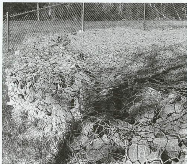
FIGURE 29 Close look at an infiltration trench and basin.
