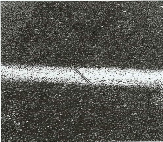
FIGURE 30 Porous pavement surface.
