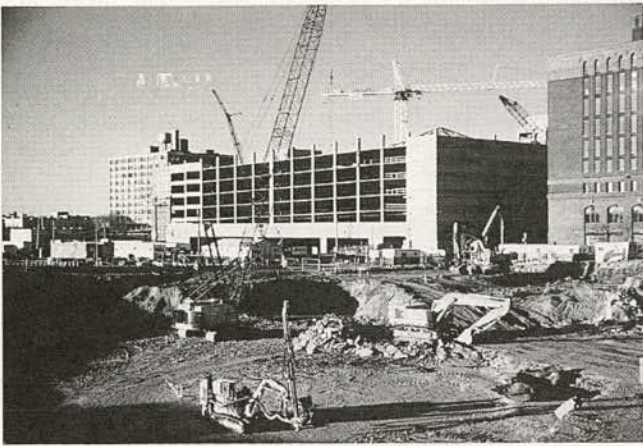
Construction of downtown parking garage for HOVs FIGURE A-6 Minneapolis HOV implementation.
