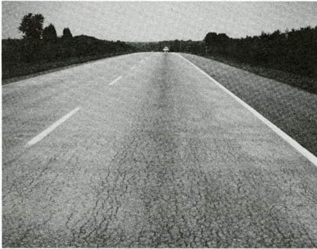
FIGURE 33 A well-defined crack pattern associated with the development of ASR in highway pavement. (Source: SHRP)
