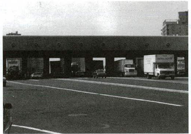
FIGURE 21b Concrete canopy, George Washington Bridge toll plaza, Fort Lee, New Jersey.
