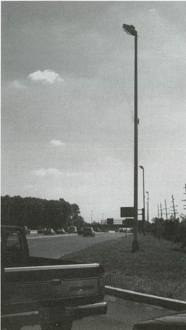
FIGURE 18b Thirty- to 35-ft (10-m) pole with offset cobra head luminaire.
