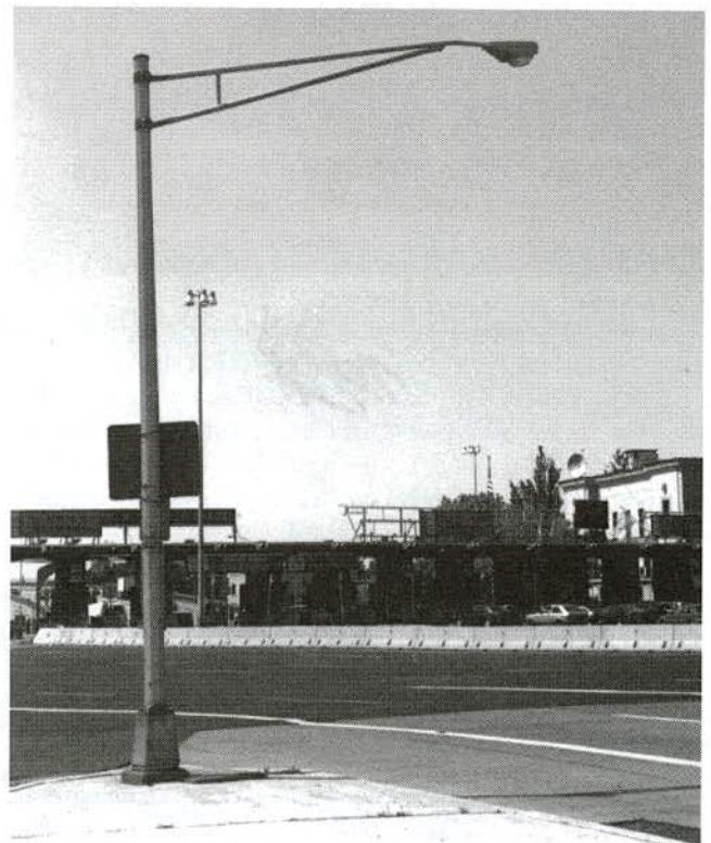
FIGURE 18a Standard mast arm with cobra-head luminaire, Benjamin Franklin Bridge toll plaza, Camden, New Jersey (Delaware River Port Authority).
