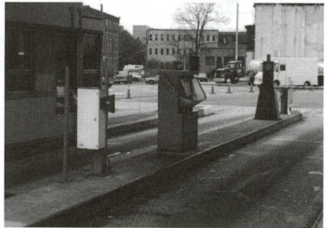
FIGURE 25c Automatic coin machine (ACM) used in conjunction with laser bar code reader and automatic gate, Benjamin Franklin Bridge toll plaza, Camden, New Jersey (Delaware River Port Authority).
