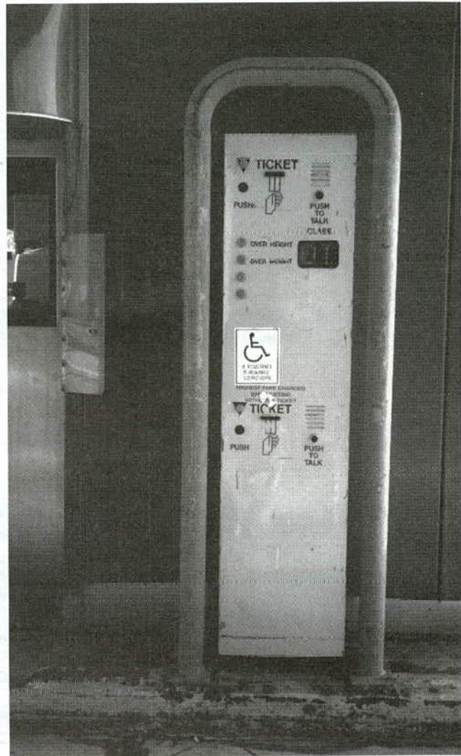
FIGURE 17b Dual-height (high and low) automatic ticket dispenser (ATD) used on the Pennsylvania Turnpike, intercom, and steel bollard used to protect dispenser (Pennsylvania Turnpike Commission).
