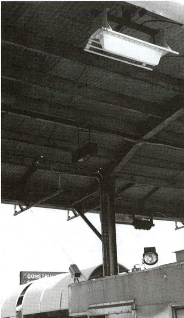
FIGURE 23c VES lane installation, E-ZPass (ETC) lane, Tappan Zee Bridge toll plaza. Note the booth-mounted camera and strobe light as well as the ETC antenna (top right) (New York State Thruway Authority).
