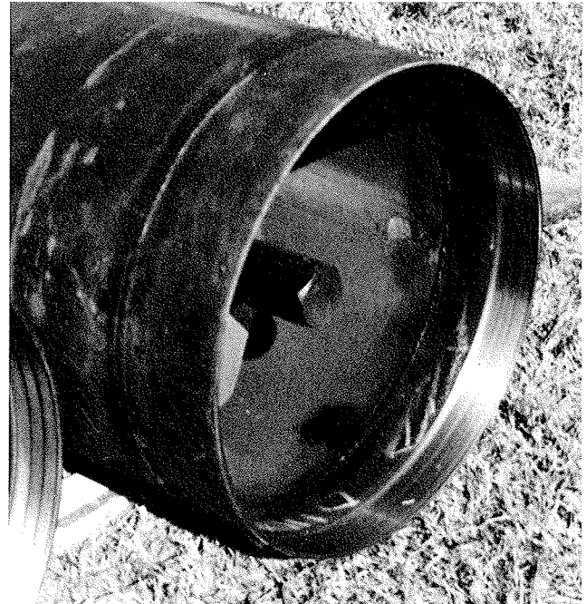
FIGURE 13 Nonweldable steel casing pipe joint.
