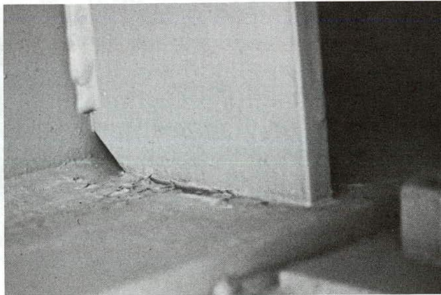
FIGURE 25 Poor paint application due to complexity.
