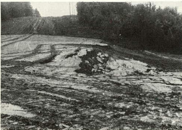
Figure 7. Embankment failure caused by placement of frozen soil (New York).
