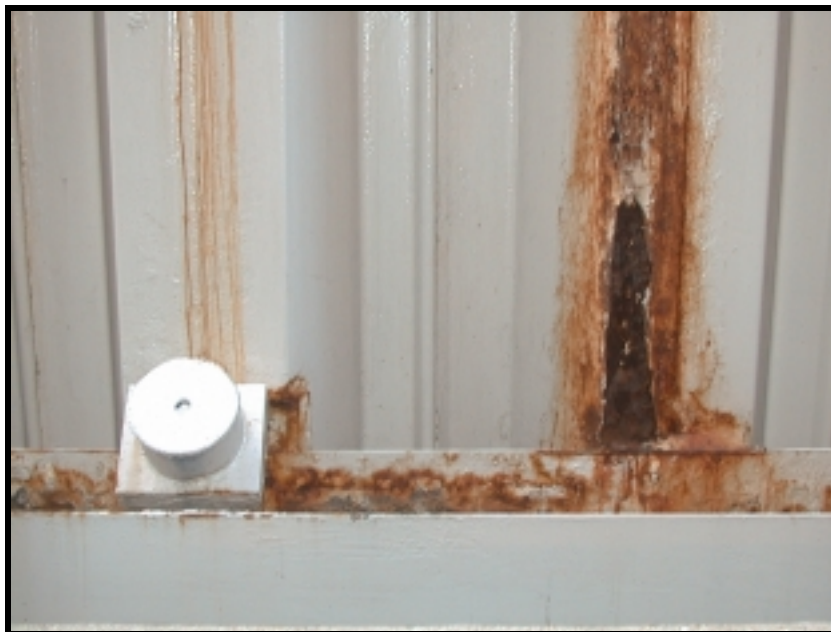
Figure 6-6: Corroded Sheet Pile Section of Anchored Wall, Pittsburgh, Pennsylvania.
