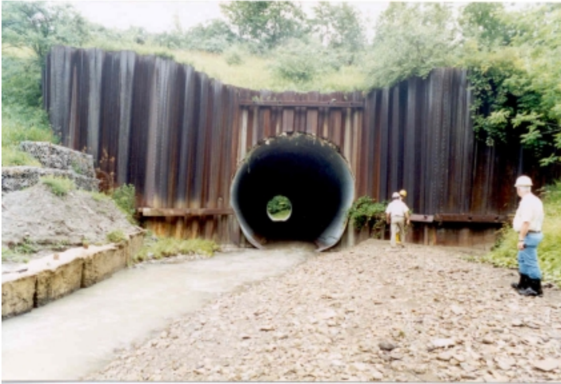
Figure 6-5: Tied-Backs Observed for Culvert Wing Wall, West Valley, NY.
