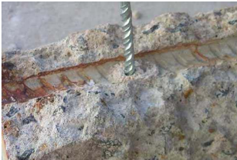
Figure A-7: Photograph of a concrete powder sample being taken by drilling at the reinforcement trace of a fractured specimen.
