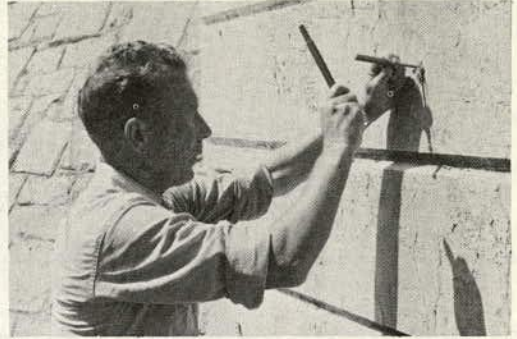
Figure 4. Setting brass insert with lead wool. This concrete is expanding at 0.03 percent per year.
