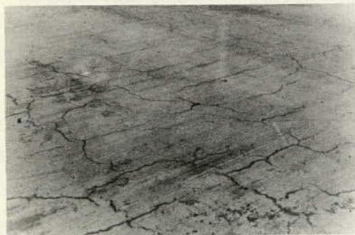
Figure 1. Random cracking in span 4 (surface damp).
