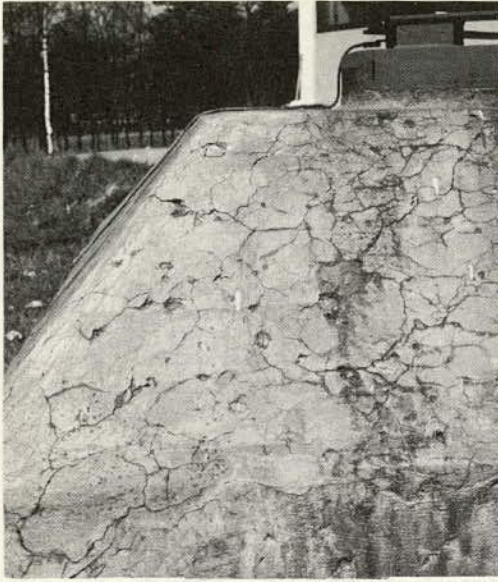
Figure 3. Close-up of mast foundation (10 in Fig. 2) showing extensive map-cracking and pop-outs.
