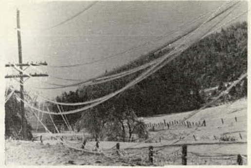
Figure 1. Downed power and telephone lines near Bradford, Vt., caused by ice loading.
