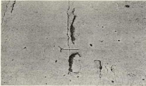
Figure 1. Typical surface spall associated with reinforcing steel.
