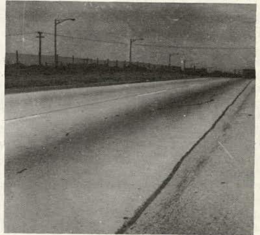
Figure 4. Longitudinal cracking with minor spalling.
