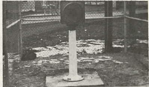
Figure 4. Skopograph projector and receiver monitors visibility at Commonwealth Edison's Dresden Power Station at Morris, Illinois.
