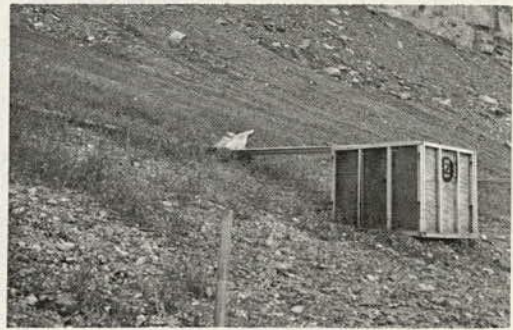
Figure 2. In demonstration No. 2, a trough of belting channels the runoff into a gutter; gutter empties into a 34.9-cu ft box.
