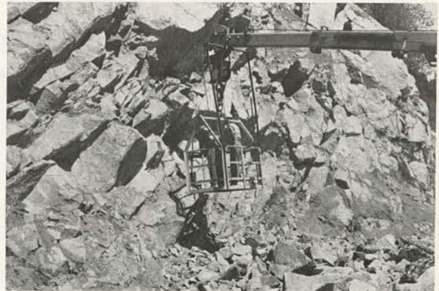
Figure 9.19. Typical hydraulic crane (giraffe) and basket used for scaling lower reaches of slopes.
