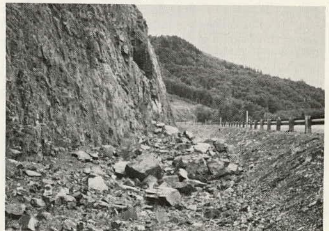
Figure 9.46. Shaped ditch to retain falling rock from nearby vertical slope on highway in Washington State (note steep slope and barrier fence on roadway side).
