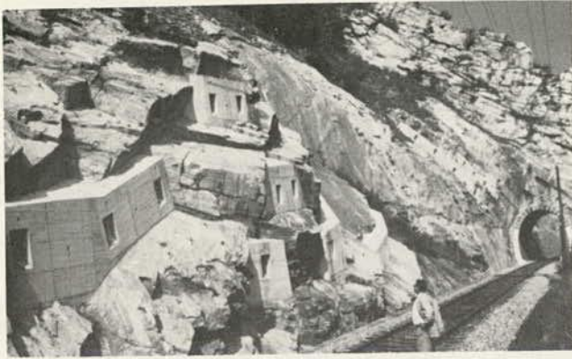
Figure 9.36. Cast-in-place reinforced concrete beams used to distribute point loads from rock bolts seated in the beams (9.84). Location is above main line of Austrian Federal Railways.
