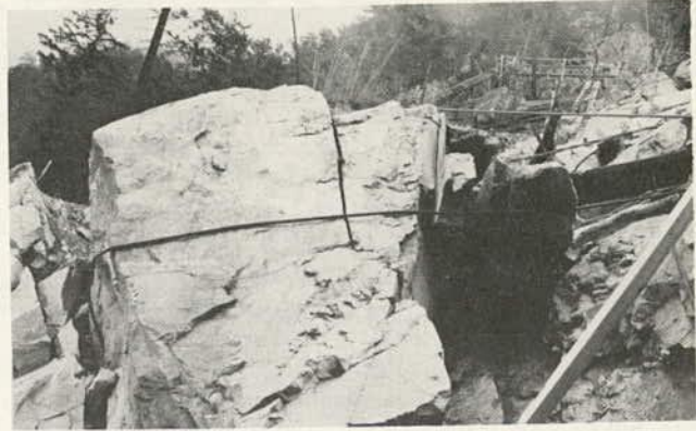
Figure 9.38. Cable lashing of a large, potentially hazardous, 2-m (6-ft) diameter block about 90 m (300 ft) above highway in Fraser Canyon, British Columbia.
