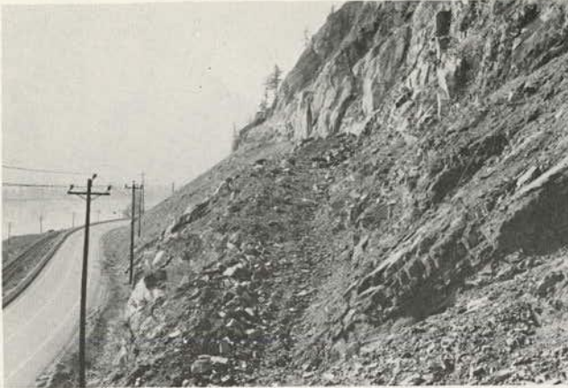
Figure 9.41. Intercepting slope ditch or cross ditch, north of Hope in Fraser Canyon, British Columbia, to catch rolling rocks originating up slope on steep rock faces (note that ditch is shaped partly in talus and makes use of blocks of rock).
