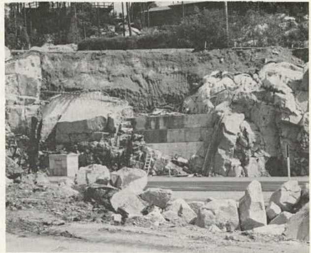
Figure 9.32. Retaining wall (top) that is partly constructed and being cast in place on sound bedrock and finished retaining wall (bottom) with stone facing. In top photo, note broad base of rock dowels that provide for added shear strength at toe of retaining wall as well as excellent bond between concrete and rock.
