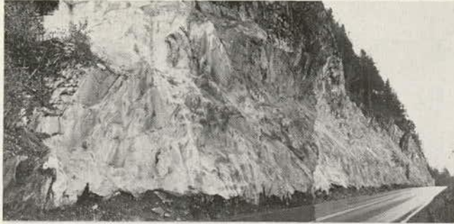
Figure 9.22. Shotcrete applied to steep high slope that is prone to minor slides and rock falls.
