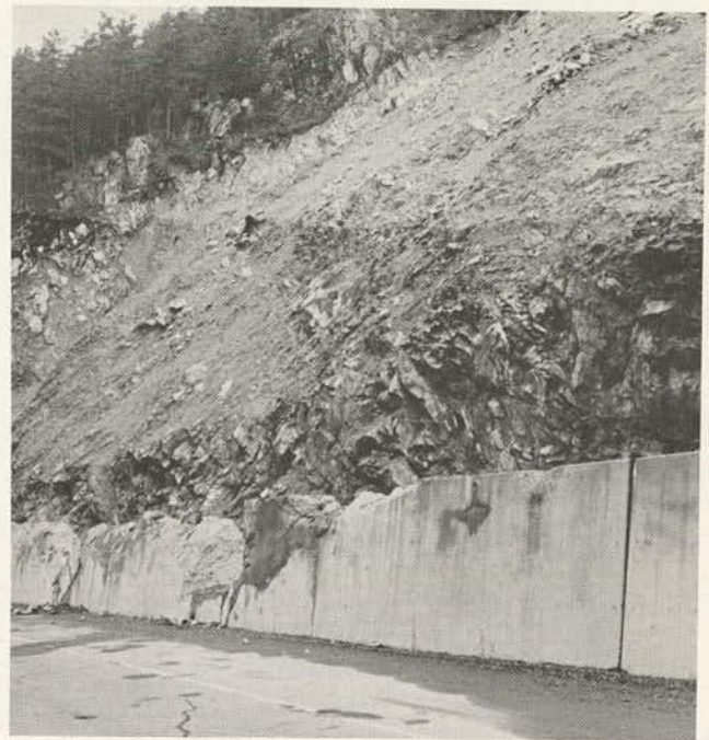
Figure 9.51. Close-up of concrete catch wall shown in Figure 9.50 (note breaks in wall due to large blocks from postglacial slide debris rolling down slope).
