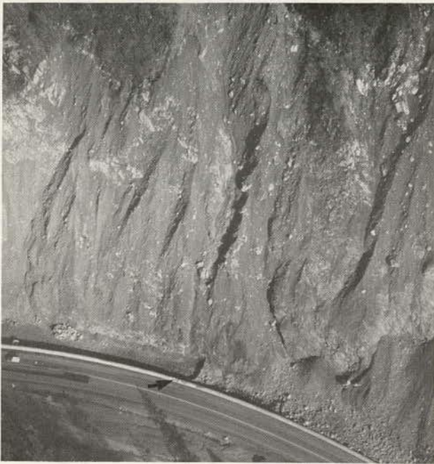
Figure 9.50. Reinforced cast-in-place concrete wall approximately 2 m (7 ft) high and 1 m (3 ft) wide across a major postglacial slide area along edge of Trans-Canada Highway in Fraser Canyon, British Columbia (note break in retaining wall where large blocks have hit wall).
