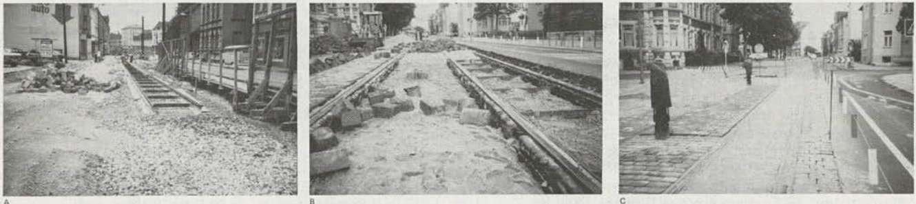
Note: A = preparation of base and assembly, welding, and alignment of track; B = placement of web fillers (hollow clay tile) and sand bed for blocks; and C = placement of blocks and cleaning and sealing of pavement.
