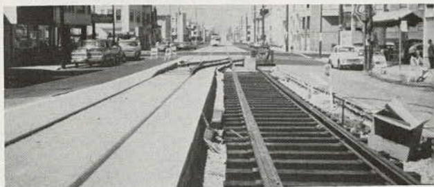
Figure 1. Construction of rigid track in San Francisco in 1975 (ballast, ties, concrete pavement).
