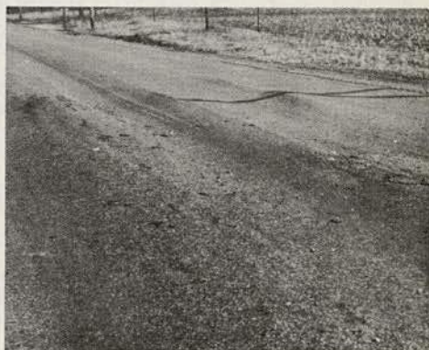
Figure 7. Subgrade Softening - Rutting - First Step in Bituminous Mat Failure.
