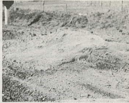
Figure 4. Frost Boil - Mud Breaking Through the Surface at the Shoulder.
