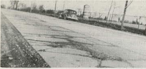
Figure 1. Pavement Broken as a Result of Differential Heaving.
