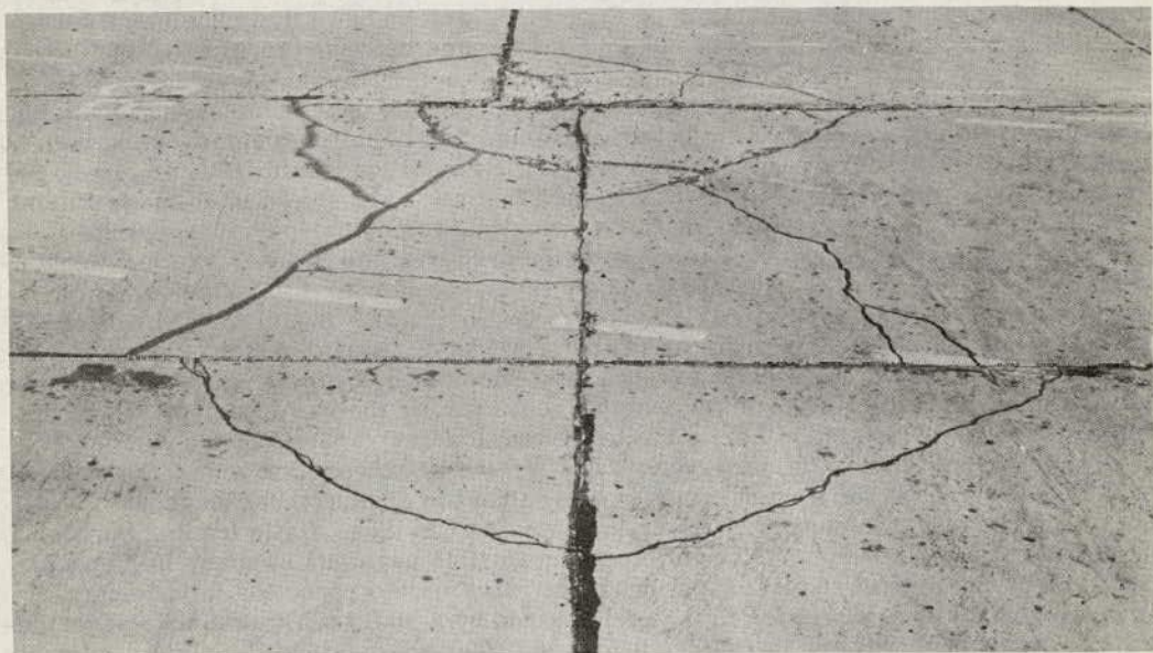
Figure 18. Condition of 7 in. Concrete Slab After 54 Coverages per Day for 15 Days and 178 Coverages per Day for 5 Days of 25,000-lb. Wheel Load (see line 65, Table 4). Pierre Airfield, Pierre, South Dakota.
