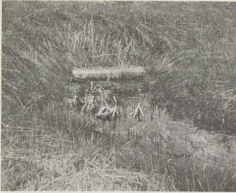
Figure 5. Tile Outlet Without Proper Outfall.
