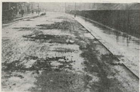
Figure 6. Damage Caused by Frost Heave in Chalk Fill.
