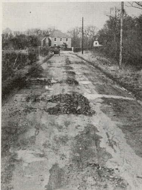
Figure 5. Frost Heave on Country Road in Southern England.
