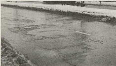
Figure 1. Surface Spalling Due to Frost (Concrete Construction).
