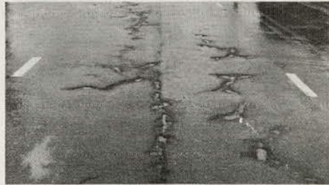
Figure 2. Separation of Two Courses of 2-Coat Asphalt Due to Frost Action.
