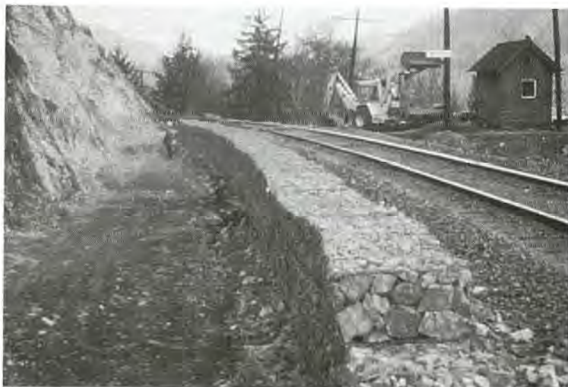
FIGURE 18-16 Rock catch ditch with 1.5-m-high gabion wall along outer edge (Wyllie and Wood 1981).
