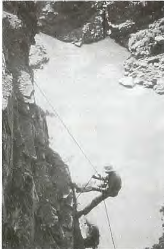
FIGURE 18-13 High scaler suspended on rope and belt while removing loose rock on steep rock slope.
