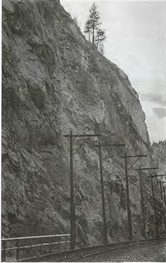
FIGURE 18-22 Typical warning fences at toe of steep rock slope to detect rock falls on railway.
