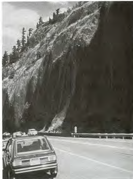
FIGURE 18-21 Wire mesh hung on vertical face to direct falling rock into ditch at toe of slope.
