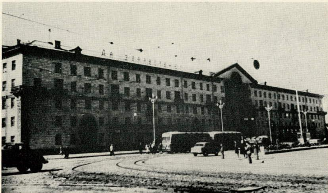
FIGURE 27 Foundations of this building in Zaporozhye showed no additional settlement when flooded with storm water.
