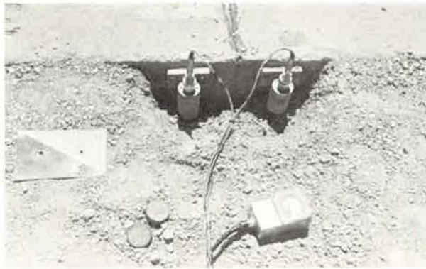
Figure 36. Instrumentation used in measurement of dynamic deflection at panel corners.
