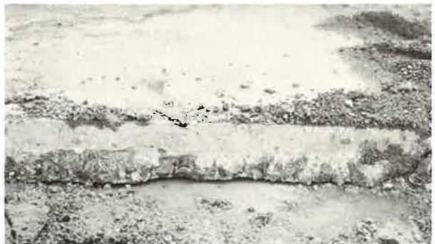
Transverse cross-section of a pumping slab showing void beneath pavement.
