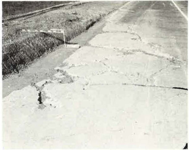
Subbase material ejected from beneath pavement overnight and deposited along edge.
