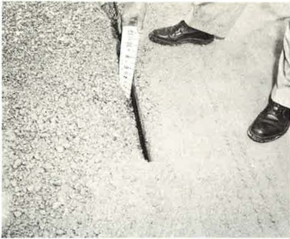
Void in shoulder through which subbase material was ejected from beneath pumping slab.
