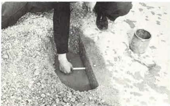
This void beneath pavement extended more than 5 ft from edge.
