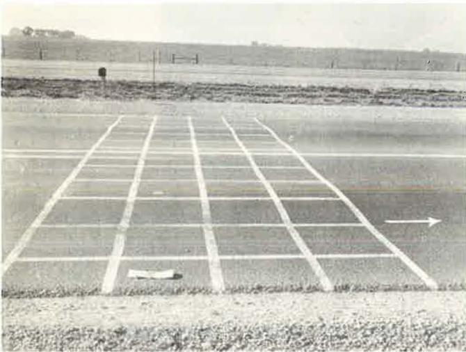
Minor rutting, slight displacement of transverse grid lines in wheelpaths.
