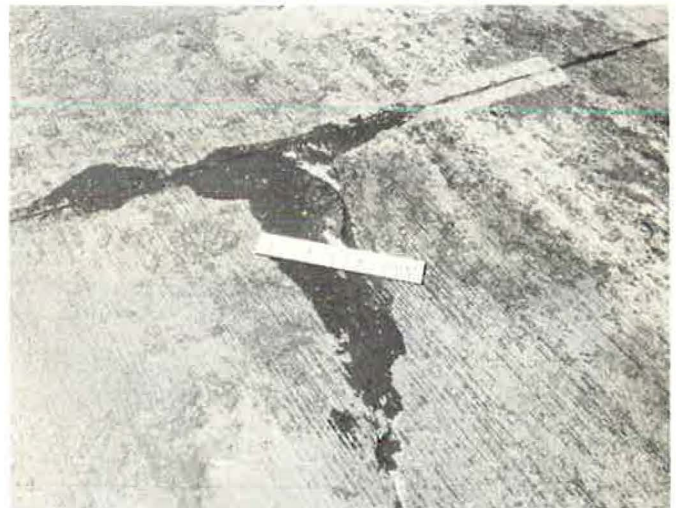
Figure 32. Examples of the four classes of cracks in rigid pavement at the Road Test: upper left, Class 1; upper right, Class 2; lower left, Class 3; lower right, Class 4. Only Class 3 and 4 cracks entered into the determination of the serviceability index.
